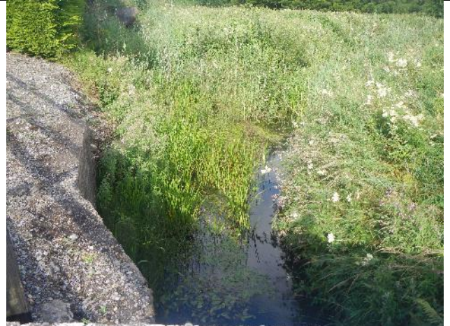
Figure 187: GI(T1) 002. Emergent vegetation choked the channels u/s of the bridge, as often occurs when a channel is dredged wider than the flow can naturally maintain.
