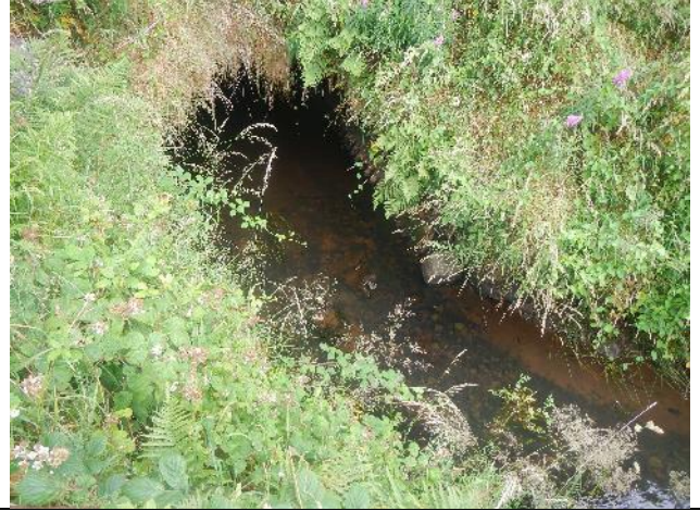
Figure 112: Sw 005 (53.944378, -8.929267). The N5 road culvert was appropriately sunken and provided free fish access. The substrate appeared to have an elevated fine sediment load, but juvenile salmonids were observed there. Further investigation of sediment sources u/s would be beneficial.
