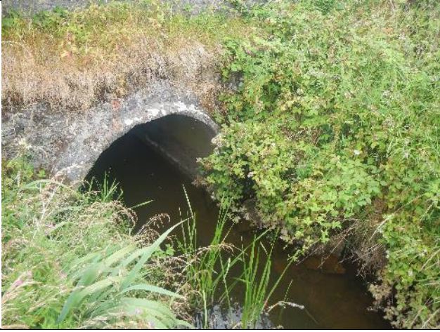
Figure 154: Ki(T1) 014. A culvert observed at the next spot-check was passable by fish.
