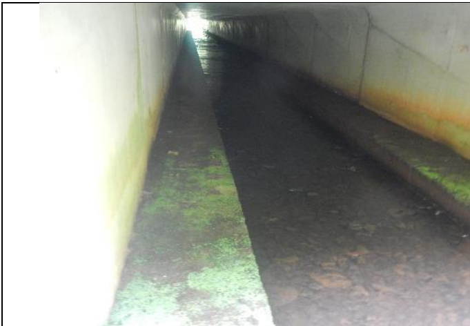
Figure 243: Gw(T1) 003. Although long, the natural substrate of R321 culvert provided reasonable fish passage
