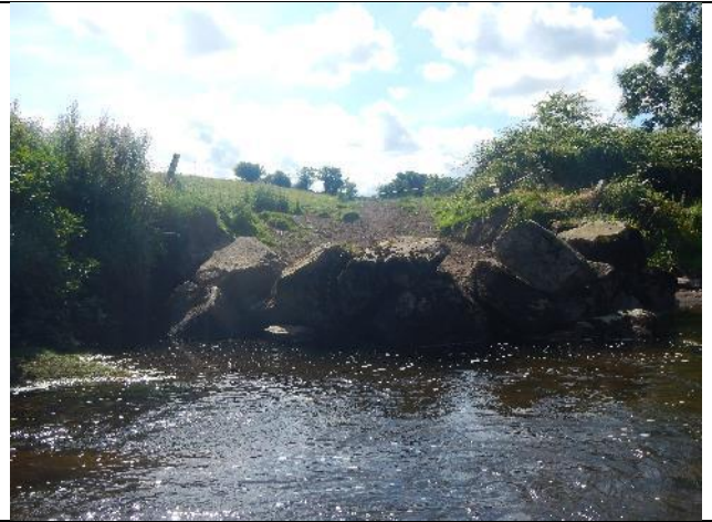
Figure 69: Mo 225 (53.931938, -9.070647). Although enclosed by boulders, this drinking bay was clearly supplying fine sediment and should be replaced with offline watering facilities.
