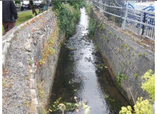
Figure 114: Sw 011. An extended section of walled channel provided poorer habitat quality, but the coarse substrate retained was still capable of supporting flow diversity and invertebrate communities, along with some juvenile salmonids. In such an artificial channel, alternate deflectors could encourage sediment retention and the formation of more discrete gravel bars.
