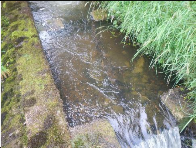
Figure 38: Mo 113. Gravel material partially infilling the pools of the fish ladder. This reduces depth and energy dissipation within the pools, thereby also reducing the ease with which fish can jump from pool to pool. The ideal solution would be to remove the old bridge and footings to allow free access to all fish in all flows.
