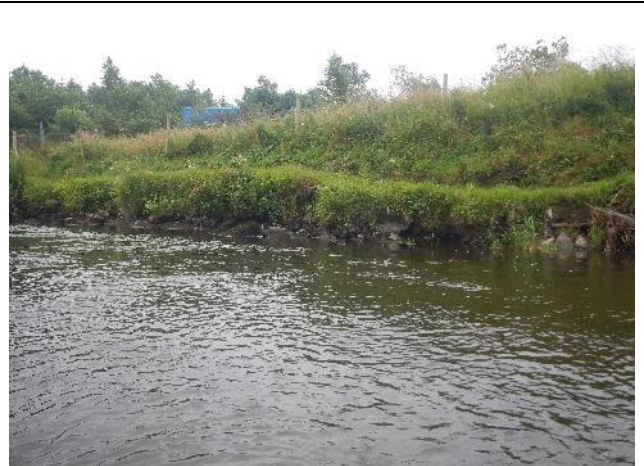
Figure 31: Mo 088 (53.948318, -9.028927). Maintaining a rougher, uncut vegetated fringe along the river side of a narrow access track would offer improved protection. Further protection could be provided with brush (live or dead) to dissipate the energy of flow hitting the bank face and/or the planting of willow whips.
