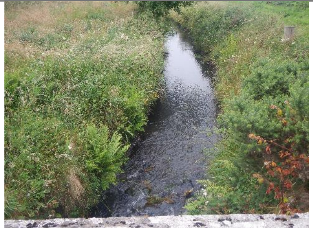
Figure 254: Tr 004. D/s of the road, raised bridge footings created a small obstruction but were rough and passable by fish. The turbulence they created gave hint of the flow diversity regular riffles and a more morphologically diverse channel should support. Lower grade land along the LB may offer the greatest potential for restoration/re-meandering but both banks have potential.
