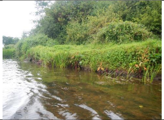
Figure 224: Gw 156 (53.906933, -9.021245). Lack of buffer fencing, reduced vegetation and increased susceptibility to bank erosion.
