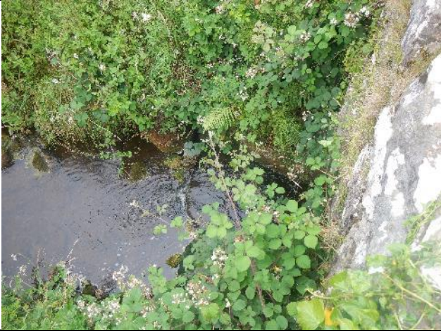
Figure 108: Mo(T1) 004 (53.945848, -9.022352). The footings of the bridge were slightly perched, but passable. They could potentially be improved with an easement.
