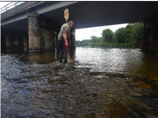
Figure 90: Mo 307 (53.93815, -9.103298). Ballylahan Bridge footings do not create a major obstruction, but they are raised and likely to create a behavioural barrier, particularly in low flow, inhibiting fish movement through the catchment. Best practice would be to have sunken the structure well below bed level. This would also prevent impounding flow u/s.
