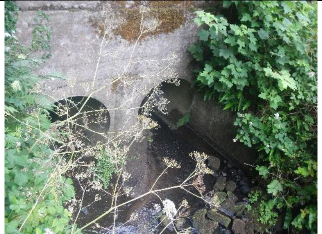
Figure 287: Ca(T2) 002. Accessibility for fish was not good owing to a pipe culvert with shallow water.
