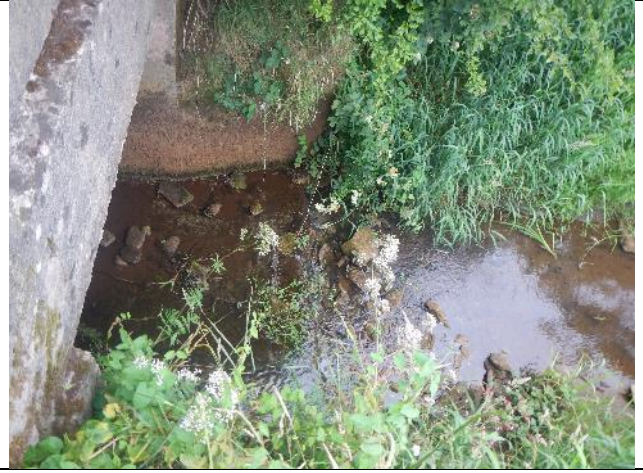
Figure 309: St(T1)10 (53.935777, -9.118007). The L715 road crossing was passable but shallow water and a step posed a small obstruction to fish passage.
