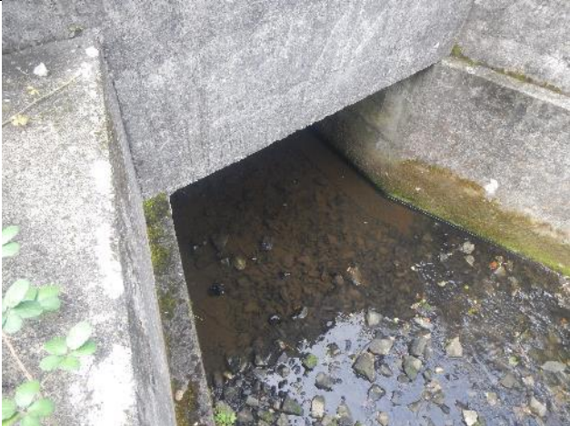
Figure 277: Ca 003. Despite being a large structure, the N5 road culvert was appropriately sunken and passable, with a somewhat natural bed.
