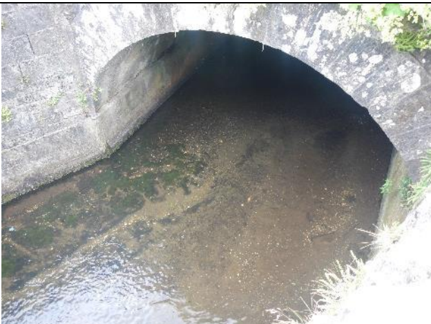
Figure 115: Sw 012 (53.945103, -8.952145). A culvert beneath the road bridge appeared passable, although detailed inspection was not undertaken. Note the fine sediment accumulation within the wider culvert channel. N.B. not all watercourse crossings around Swinford were inspected, so others may pose obstructions.
