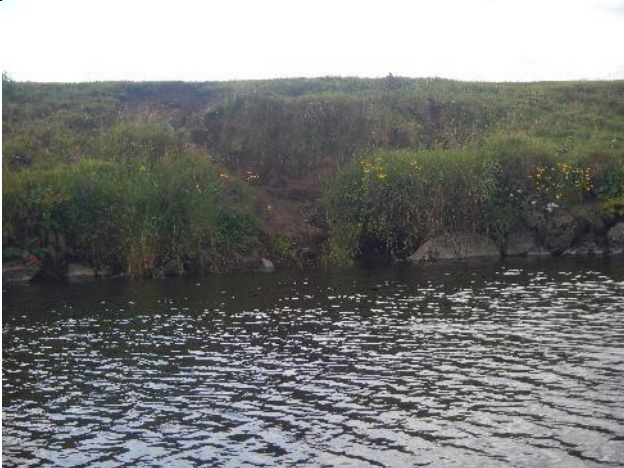
Figure 100: Mo 336 (53.945288, -9.122455). At one of the few sections where livestock had access to the main riverbank, vegetation was denuded, and erosion and fine sediment input were occurring.
