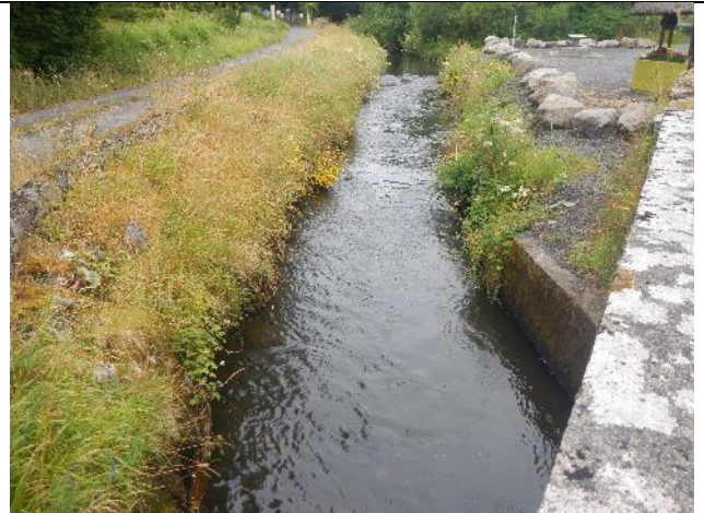
Figure 260: Tr 023. D/s of the village, the channel was still significantly modified, but had begun to improve naturally, with depositional features diversifying the bed and healthy bankside vegetation. The habitat continued to improve d/s. Numerous juvenile salmonids were observed u/s and d/s, demonstrating the potential value of this tributary.
