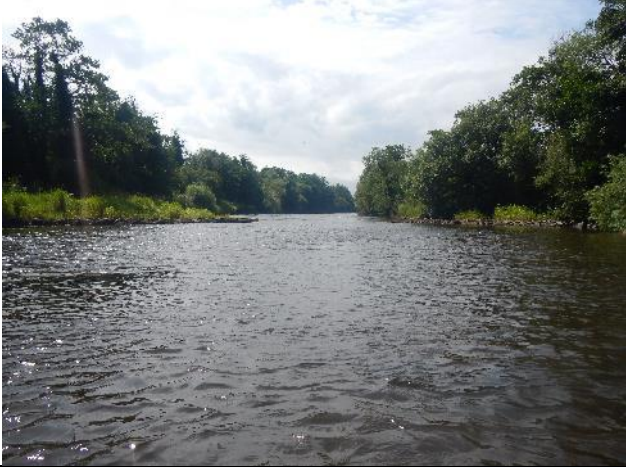
Figure 50: Mo 169 (53.9372, -9.04782). Two sets of paired groynes in a long straight channel section were inhibiting natural channel recovery by focussing flow down the centre of the channel.
