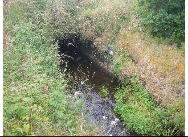
Figure 126: Sp 007 (53.927365, -8.95989). The road culvert appeared to be appropriately sunken and passable by fish.
