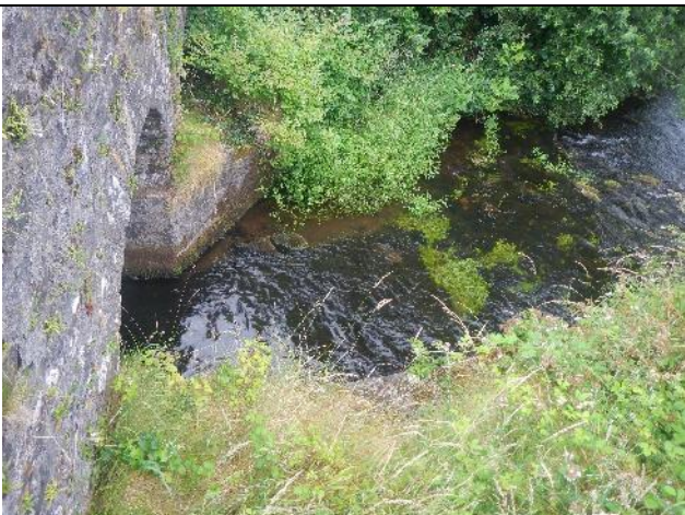
Figure 127: Sp 010 (53.928007, -8.960362). An older bridge just d/s also appeared passable, but the narrow aperture was accelerating flow velocities.
