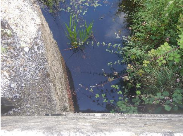
Figure 186: GI(T1) 001 (53.80036, -8.744247). At the u/s spot-check on the Glore tributary, the channel was overcapacity with little flow diversity, but the culvert appeared to be passable by fish.
