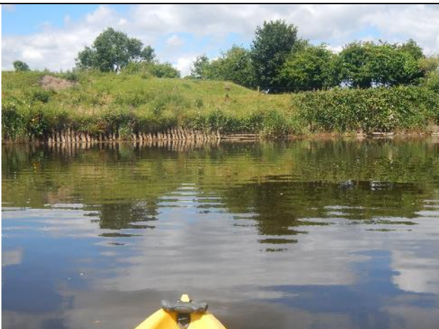
Figure 96: Mo 325 (53.940722, -9.119825). Log piling of the LB. This is counterproductive as the hard, immobile feature will simply deflect erosive forces to the adjacent bed and bank. Moreover, the prevention of tree and vegetation growth among the bank face means that when it fails, there will be nothing to hold the bank together (unlike a naturally well-vegetated bank).
