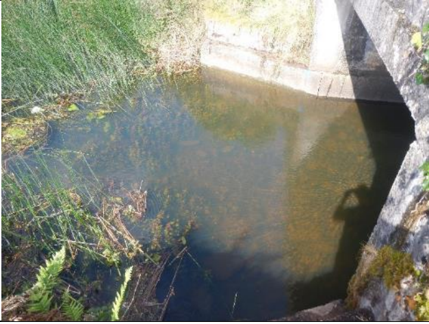
Figure 163: GI 027 (53.813167, -8.837828). D/s of the road bridge, the channel was partially choked with vegetation, but note the lack of excess algae (also see d/s - Figure 166 - where algae is a significant issue).
