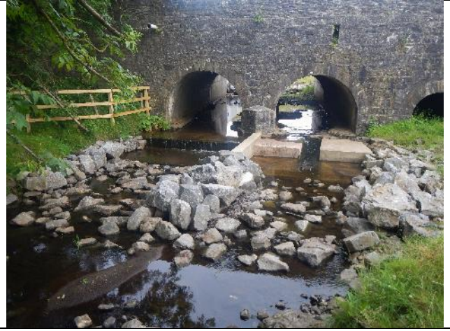
Figure 317: LiSt 017 (53.892908, -9.110955). Recent work at the N5 bridge footings may afford some fish passage but could have been fish friendlier if the rock armouring had simply been finished to the height above that of the footings. Access was not possible d/s, but increased sinuosity in the lower reaches may offer improved habitat quality worthy of further investigation.
