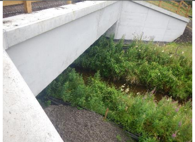
Figure 120: Sw 026. The N26 road bridge was clear-span, creating minimal impact upon the river and no issues for fish passage.
