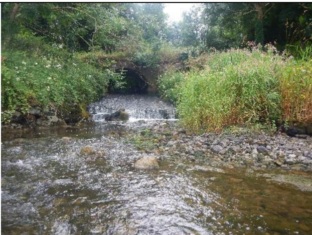
Figure 36: Mo 106 (53.945018, -9.03295). Two access routes exist to the Spaddagh, the first via perched bridge footings that are impassable in most flows but may attract and delay fish. Note the gravel deposition, which is likely to at least in part be material supplied by the Spaddagh.
