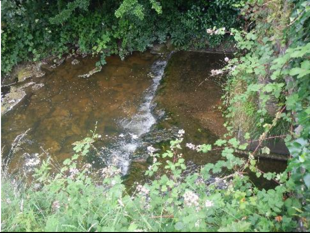
Figure 148: Ki 030 (53.928437, -9.022557). The footings of the furthest d/s road crossing created a small obstruction. However, a series of three boulder weirs/pre-barrages d/s may well be an attempt to ease a bigger step and fish passage issue, probably created by the dredging and lowering of the Moy. Baffles could slow and deepen flow over the footings to ease passage.
