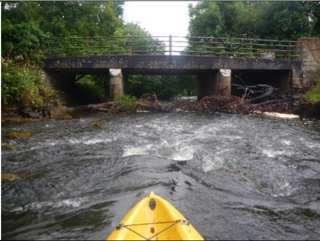
Figure 211: Gw 098 (53.8873, -9.007168). Debris at the L1919 road bridge may elevate flood risk somewhat but posed no real issue for fish passage.
